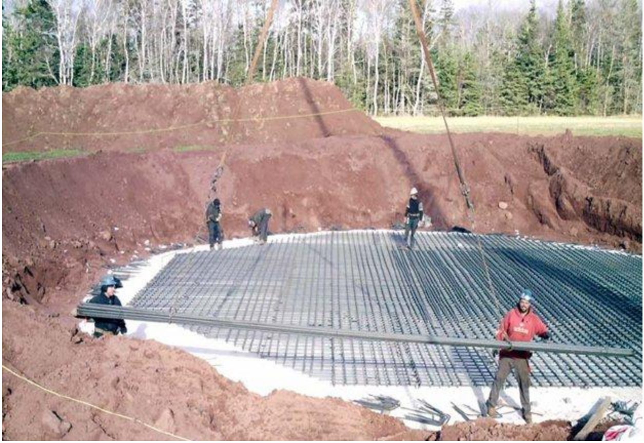
The base of one industrial turbine. Thousands of tonnes of concrete must be poured in order to hold the wind turbine up.
